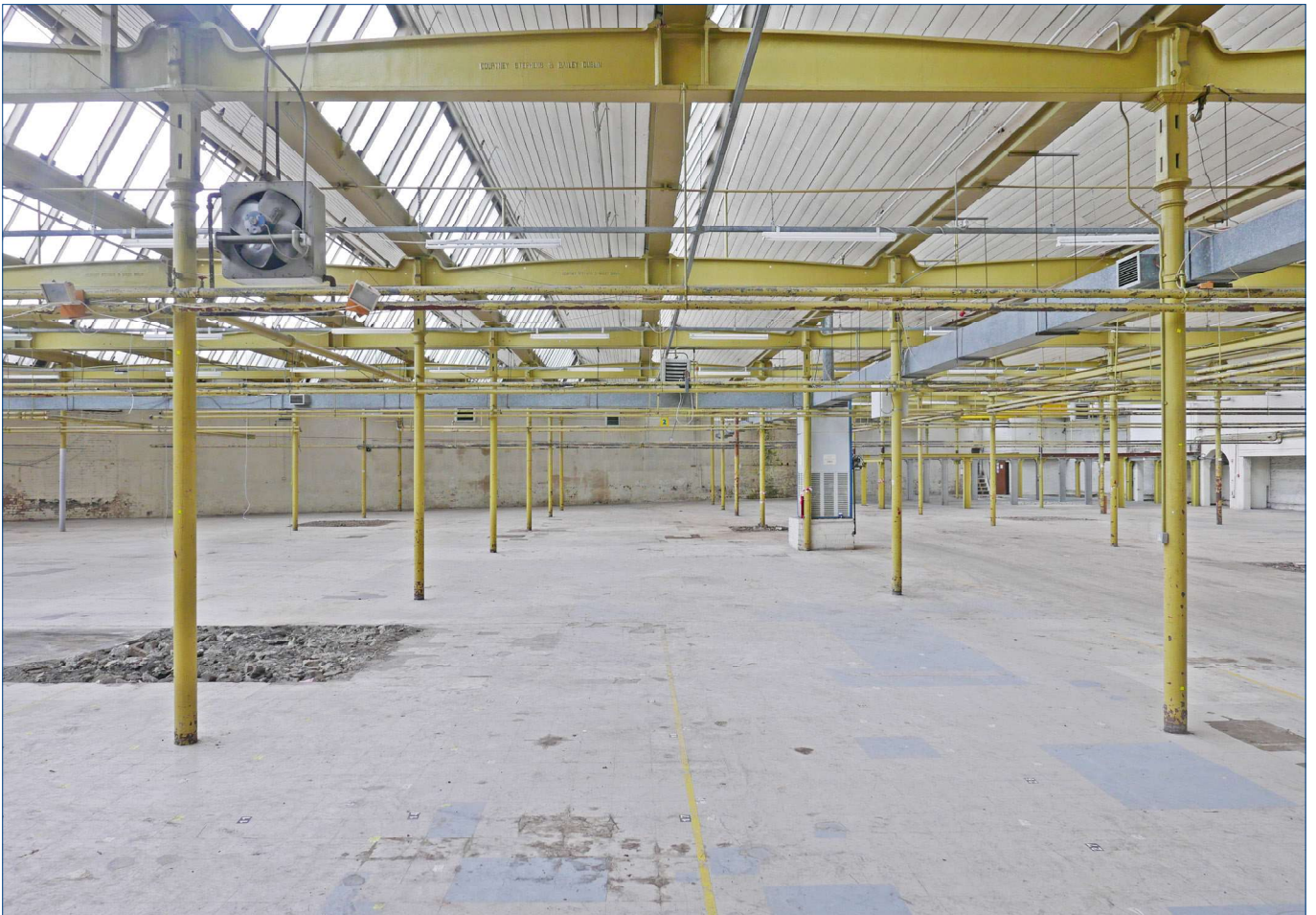
General view of the warehouse looking east, showing the columns the main beams supported by the columns and running north-south and the gutter-beams supported on the ends and centre of the main beams and running east-west
