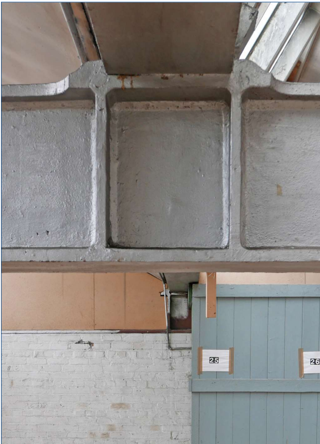
Detail of the centre of one of the main beams showing the recess to take the gutter beam above. The gutter beams join over the main beams and there is some evidence of rust from water penetration seen at the top of the main beam.
