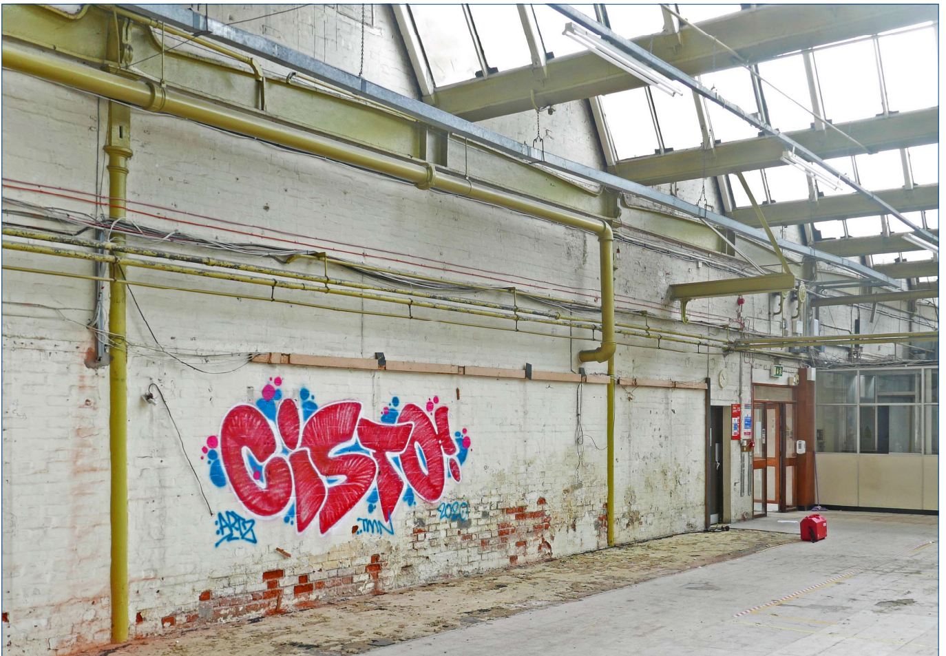
View of part of the west wall of the warehouse, showing both columns and beams embedded in the wall.
