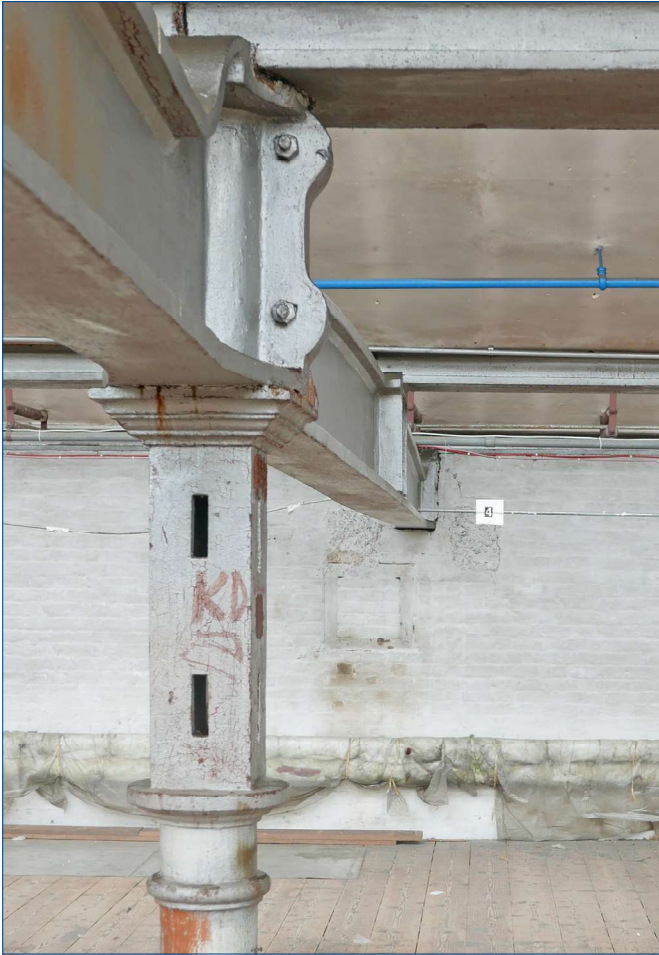
Detail of the top of a column and the joint between two main beams above, showing how the ends of the beams are bolted together.
