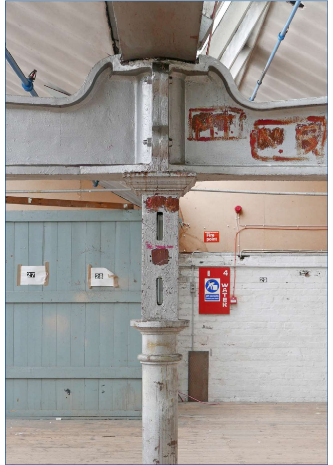
Detail of the top of a column and the joint between two main beams above, showing a gutter beam resting into a recess in the top of the beams
