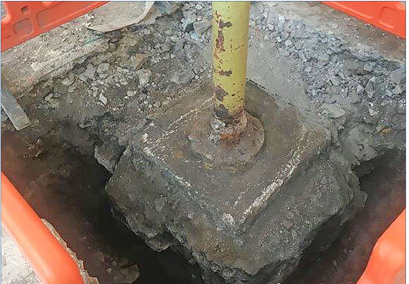
View of a trial pit excavated to show the detail of the base of a column. The base of the column flares out to produce a broad flange to spread the load. Under the column is what appears to be a granite slab some 750 mm square.
