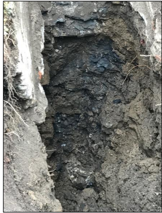
Plate 4 Mudstone at base of quay wall
