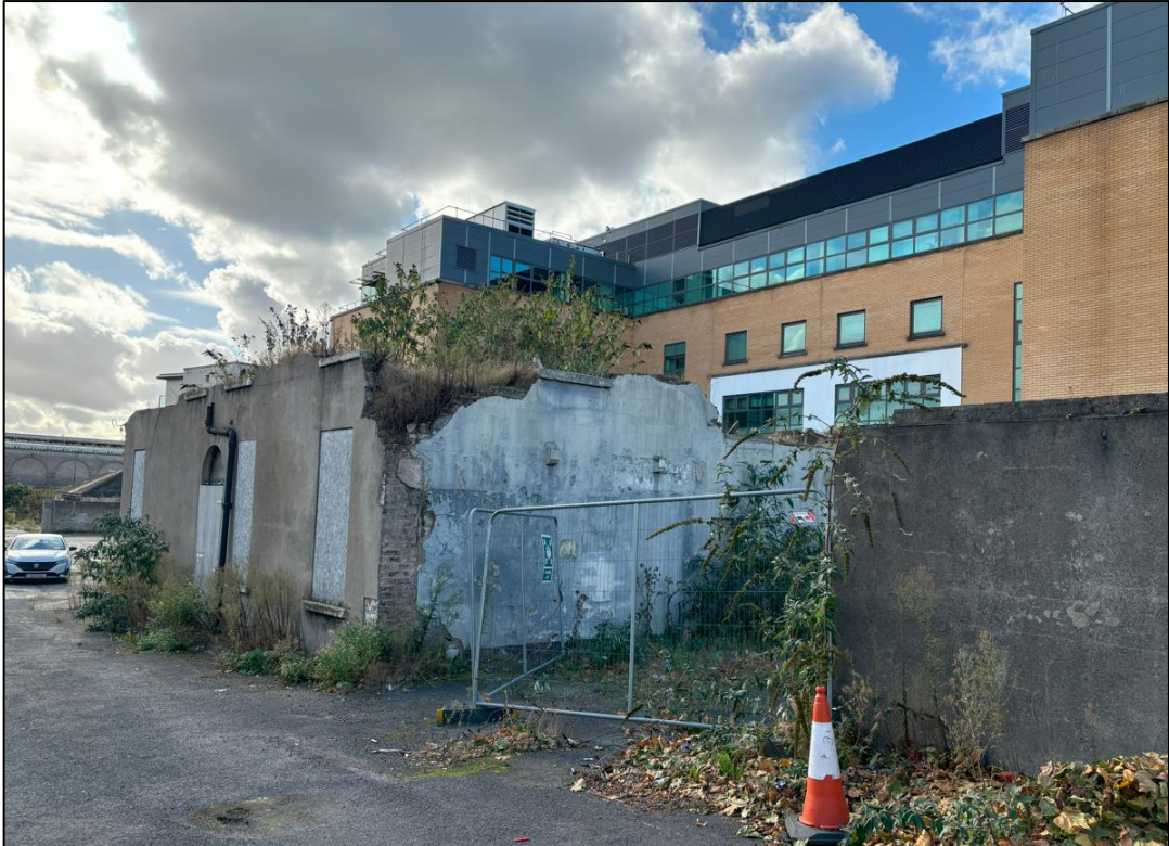
Plate 3 Part-demolished 19 th century house, facing SW, with new development overlooking to rear
