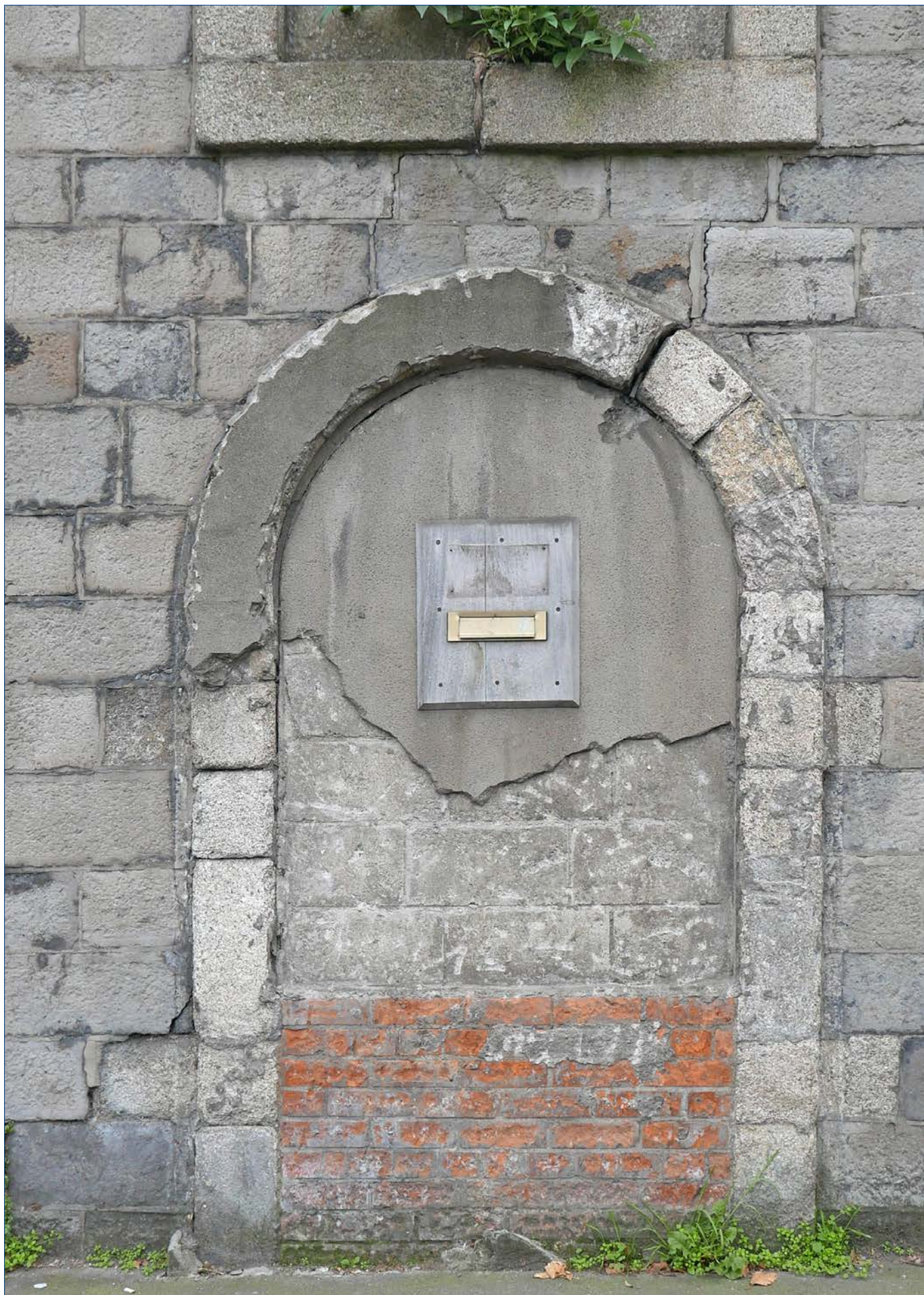
Arched side entrance in the eastern flank wall to the gateway. Perished granite stonework can be seen where areas of render has been stripped off. Originally there may have been a round headed doorway, a window opening, or possibly simply a recessed panel.
