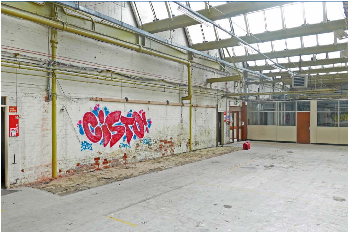
View in the Warehouse looking towards the north west corner. The 24 foot cast iron beams bear the name 'Courtney Stephens & Bailey'. These beams in turn support cast iron gutters spanning 12 feet that support the 'northlight' roof. It has not been possible to establish the origin of the columns supporting the roof beams.
