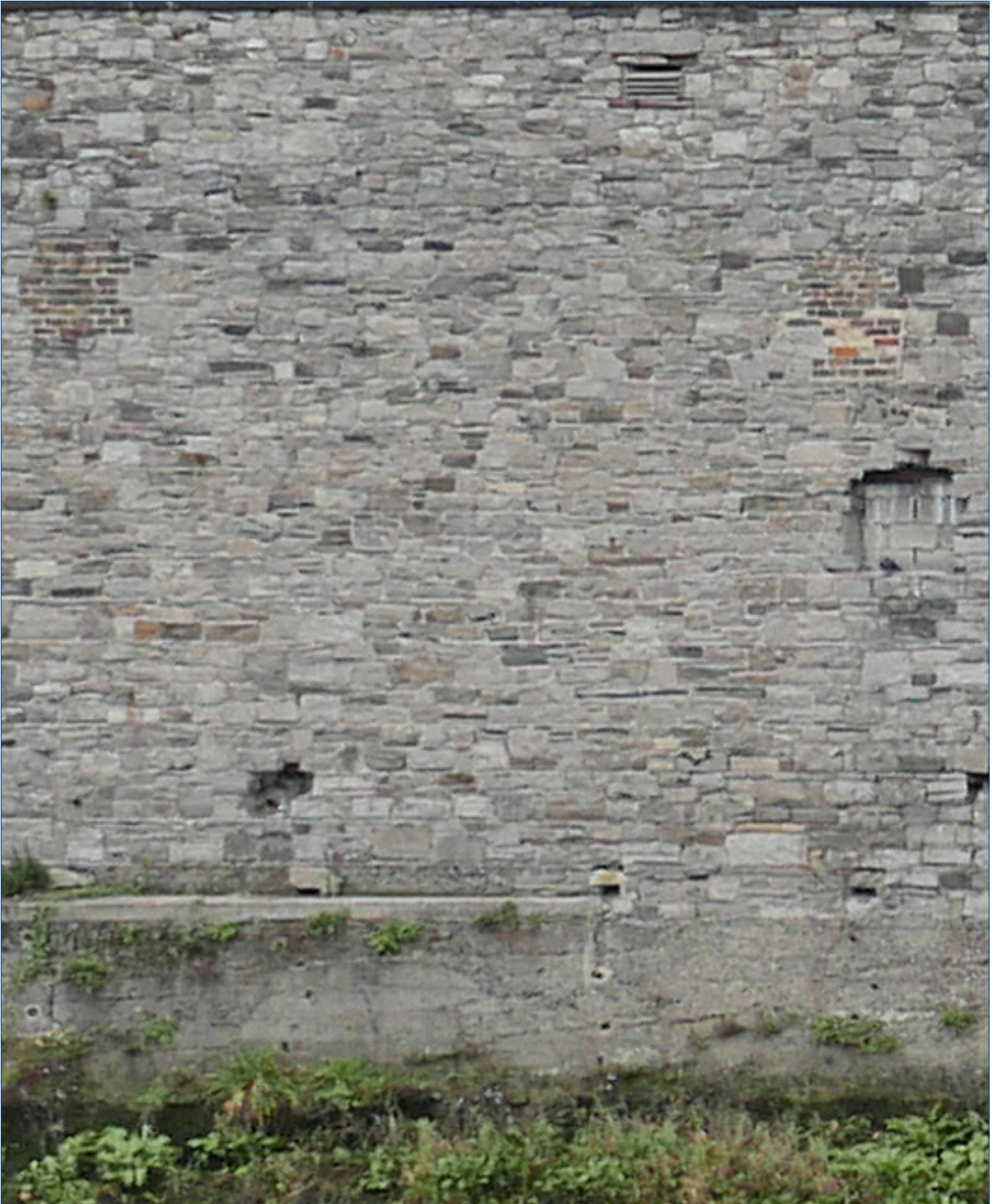
Close-up view of part of the Riverside Stone Wall. The wall is constructed of limestone in a coursed rubble pattern. The courses (dayworks) appear to range in height from 375mm to 400mm. This is less than the more normal 460mm (18 inches) and could suggest that the stone is second hand coming from former buildings on the site. The stonework pattern is less regular towards the top of the wall, and the stones near the top of the wall are smaller.
