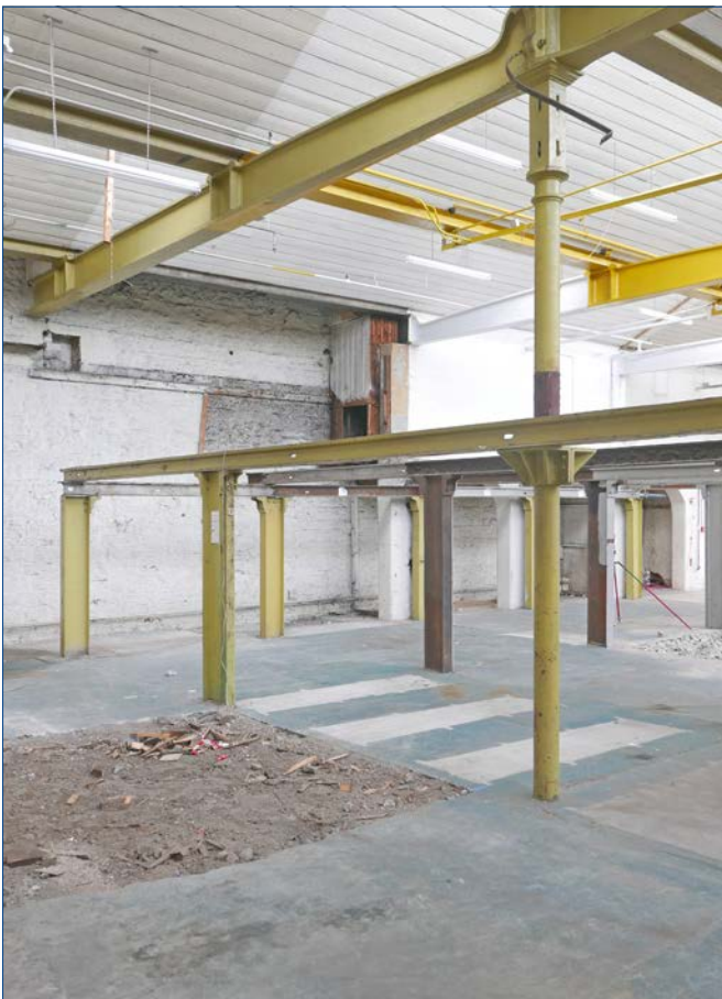
Mezzanine structure near the south west corner of the Warehouse. One of the main columns is seen with a collar supporting two lengths of tram track passing at right angles. One special extended main roof beam continues to the external Riverside Wall
