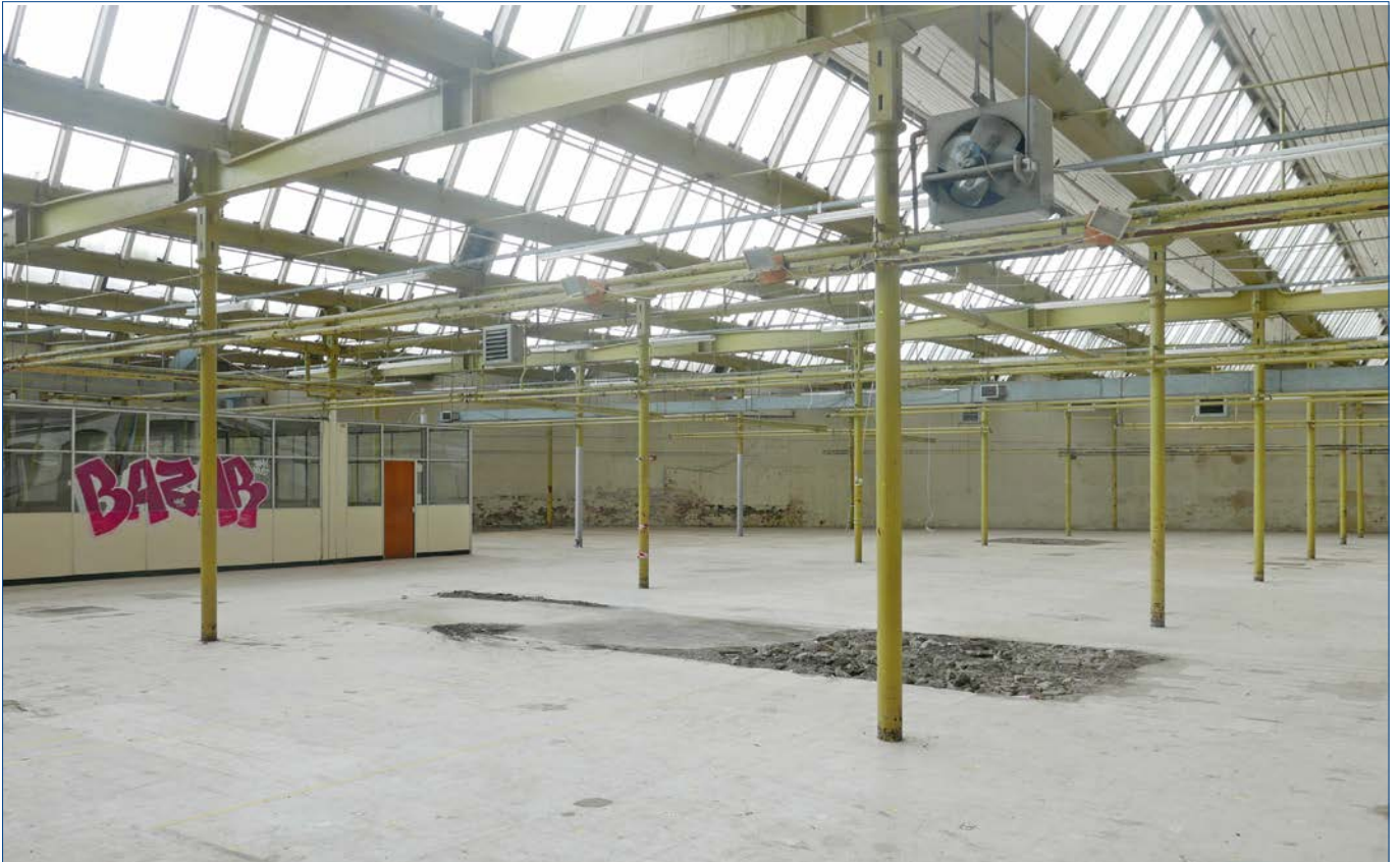
View looking west from the centre of the main Warehouse. The Warehouse is roughly triangular on plan. On the southern side, there is an inner brick wall, parallel to but not as long as the Riverside Stone Wall. On the east side, and curving around to the north, there is high grey painted brick wall along Parkgate Street. To the west and north there are also brick walls. The surrounding brick walls support the ends of the cast iron beams and gutters.
