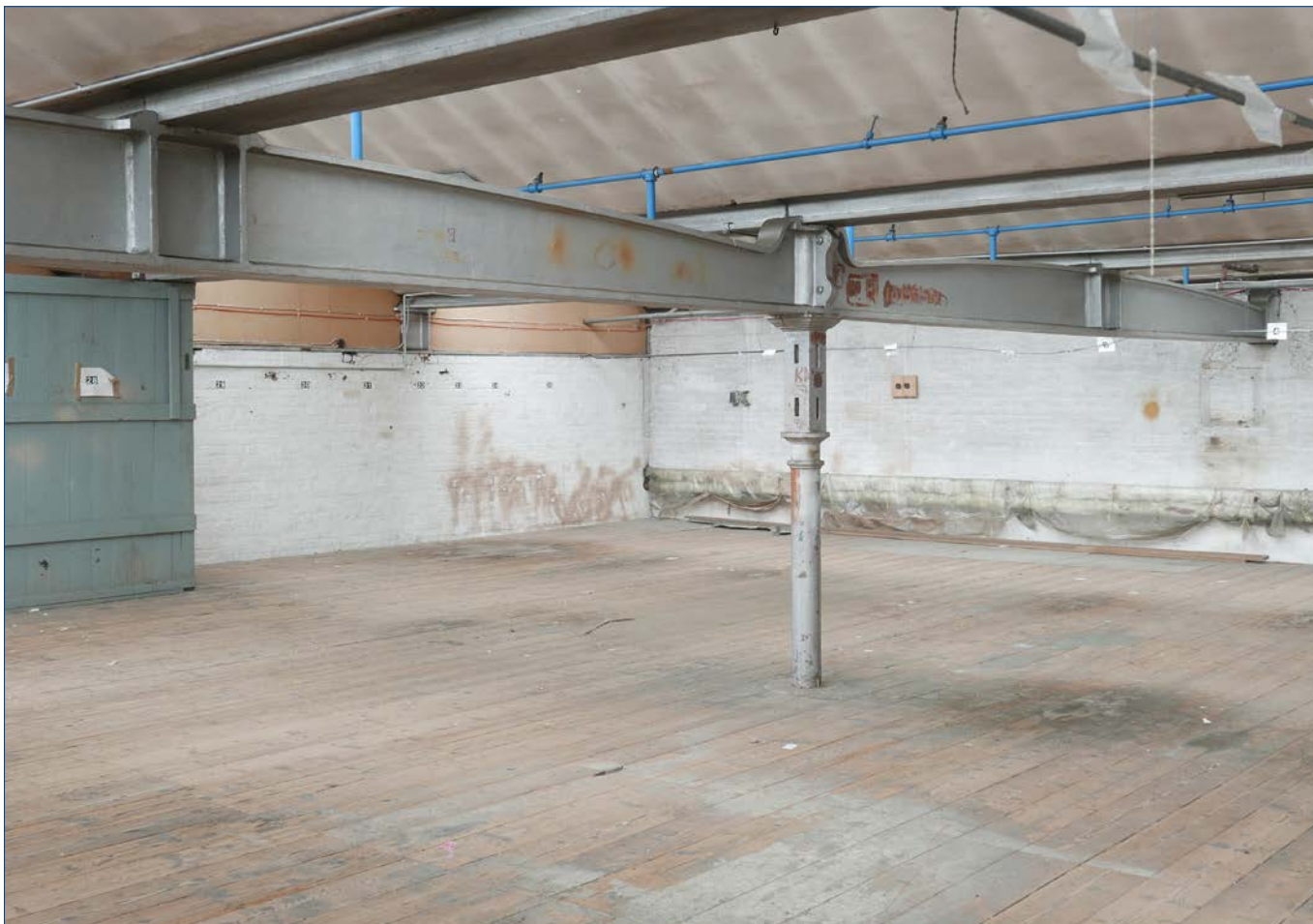
Mezzanine level in the south west corner of the Large Main Warehouse.
