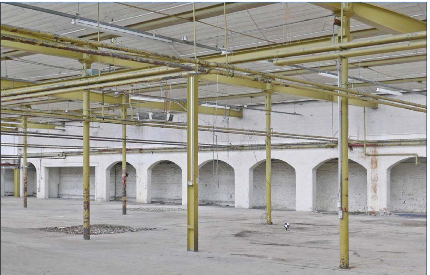
View in the Warehouse, looking south towards the arches of the separate inner brick wall. In all but two cases, the cast iron beams supporting the roof stop at the inner wall and do not continue to the Riverside Stone Wall.
