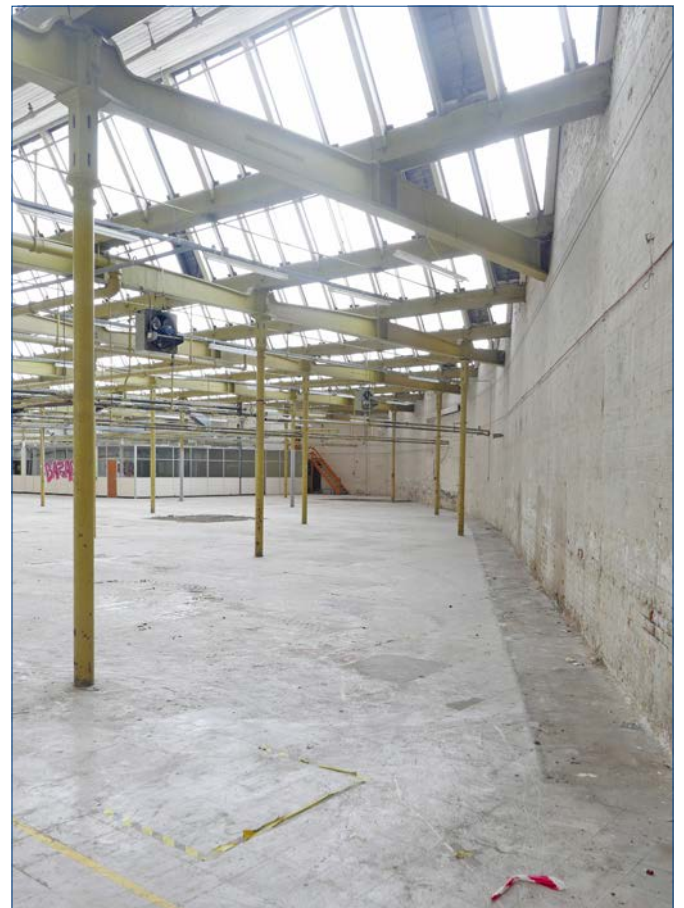
View of the interior of the large warehouse, looking north west. The curved brick wall to facing onto Parkgate Street is seen to the right, with cut back cast iron roof beams built into the wall.
