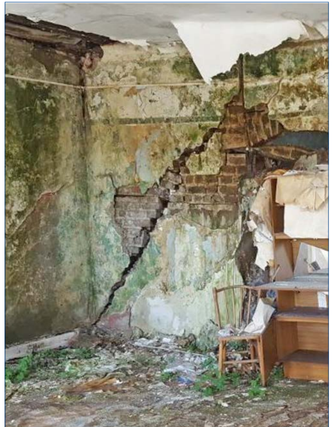
Interior view of 'Kingsbridge House' showing the structural failure of an internal spine wall. This image is from a report dated September 2016 by DBFL Consulting Engineers.
