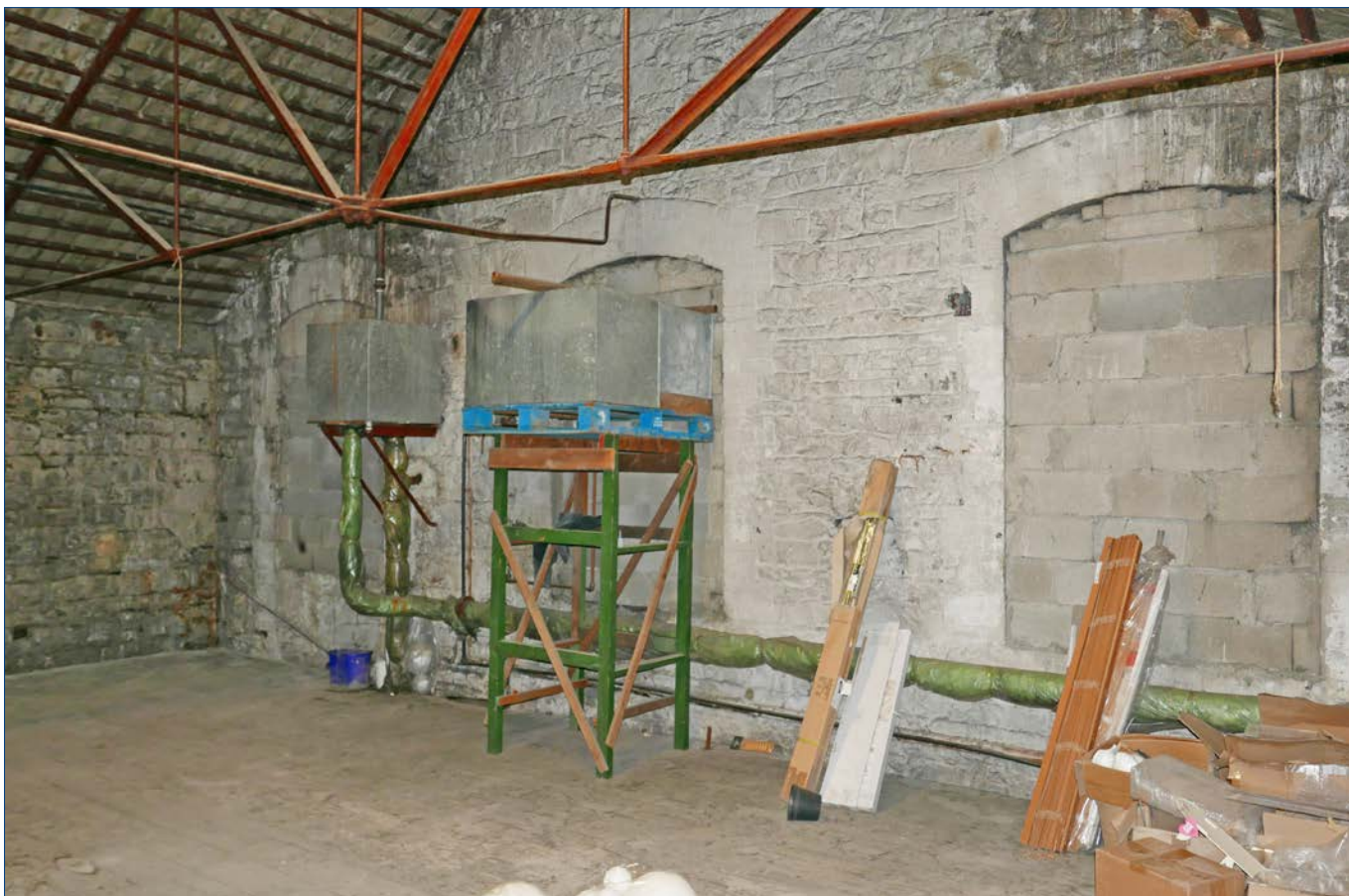
Large gabled building • upper floor • space at the north end of the building, looking north west.
