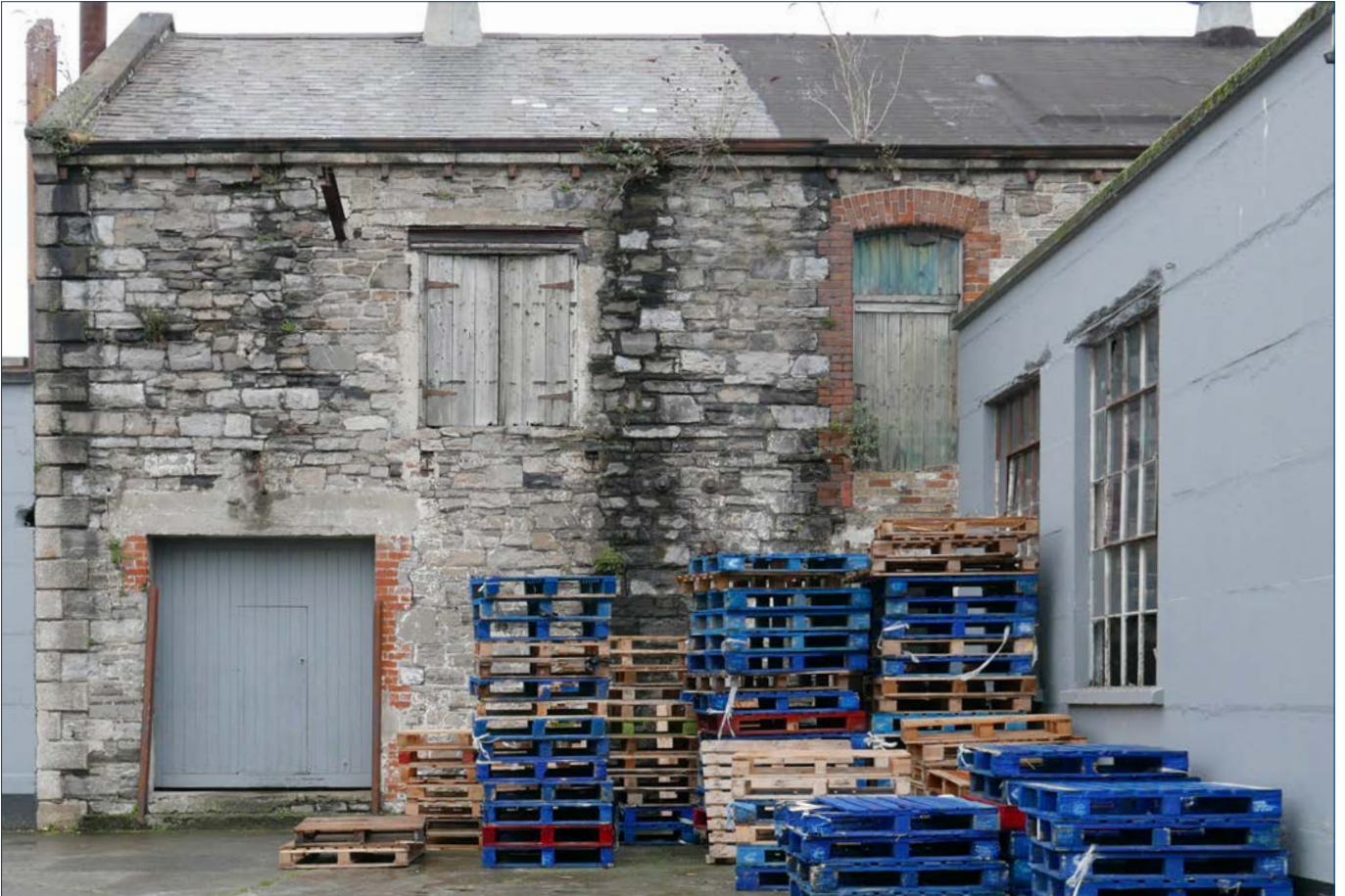
Large gabled building • north end of the west facade. Of the three openings seen in this view, only the opening to the right, with the brick trim, appears original.. The stonework is in need of cleaning, repair and repair of pointing. The slated roof needs to be repaired and reinstated.
