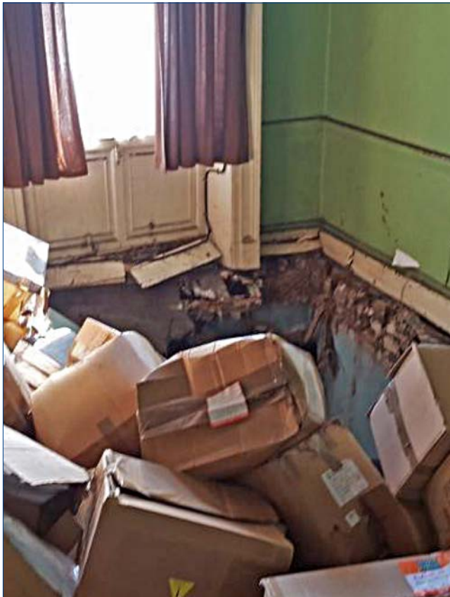
Interior view of 'Kingsbridge House' showing the ground floor partially collapsed into the basement. This image is from a report dated September 2016 by DBFL Consulting Engineers.
