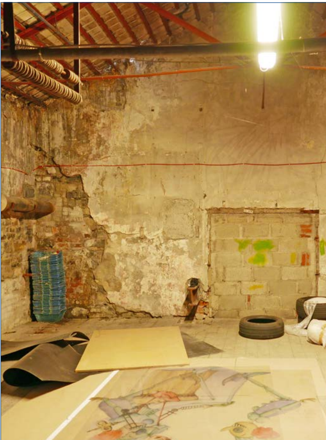
First floor space in the small gabled building looking south towards the River..
