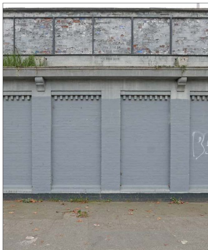
Typical bay of the wall of the warehouse facing onto Parkgate Street. Granite corbels carrying a moulded cast iron gutter with cast iron gutter beams over
