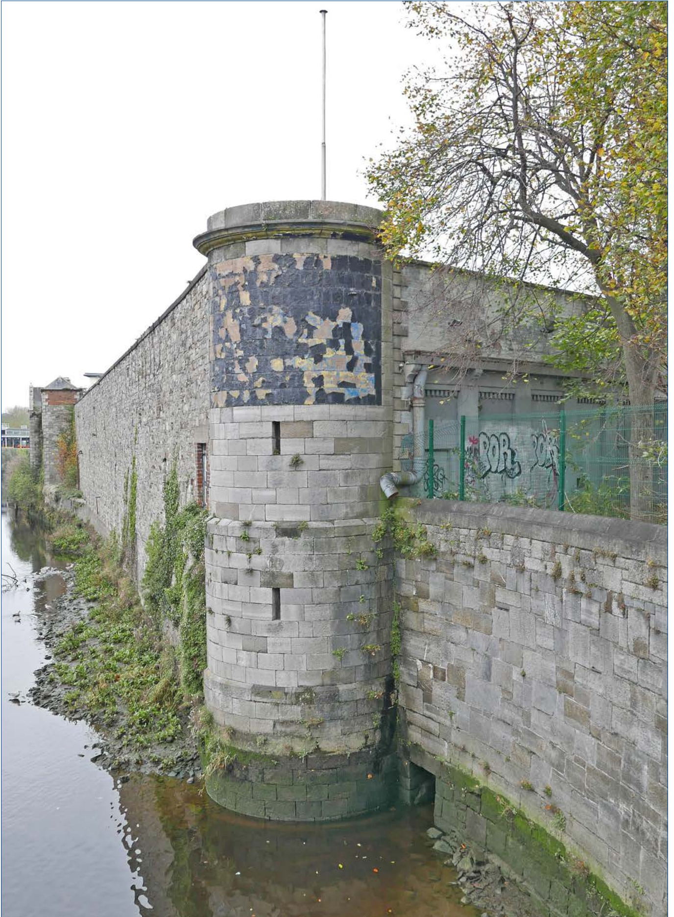
The turret is constructed in the main of cut limestone in an ashlar pattern. The cornice and blocking course are in granite. The Turret appears visually to be in relatively good condition though there is a need for some careful non-aggressive stone cleaning, removal of plants, and minor stone and pointing repair. The opening in the flank wall near the foot of the Turret is where the Viceregal Stream enters the River Liffey
