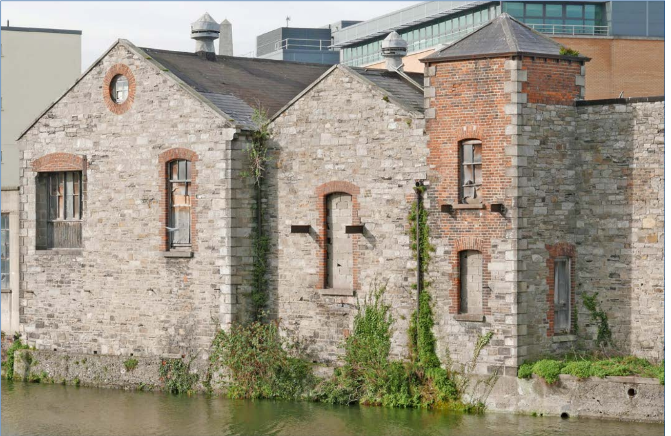
Oblique view of the river buildings, looking north west. The shape of the shadow of the square tower on the river wall suggests that the upper half of the river wall tilts back at that point. There is an opening on the east side of the Square Tower, a former door or window. It is proposed to fit a simple modern window into this opening.
